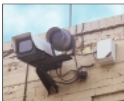
CCTV camera protected from a direct lightning strike, by one of the building's 'lightning conductors', and from transient overvoltages by protectors in a WBX 4/GS secure enclosure.
