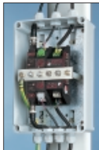
Protectors for the video (ESP CCTV/B, left), camera telemetry (ESP 15E, centre) and the low current mains power (ESP 240-5A, right) inputs to a camera, installed together on a CME 4 mounting and earthing kit. Note that the protectors have been cross bonded to the metal work of the pole (out of shot).
