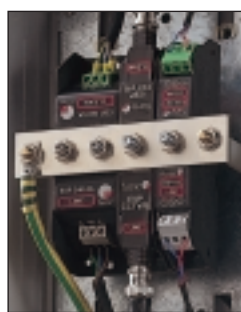
To protect an outside CCTV camera, protection on the power supply (here an ESP 240-5A) is installed alongside video and telemetry line protection, on a CME 4 (mounting and earthing kit), inside a WBX 4/GS enclosure.
