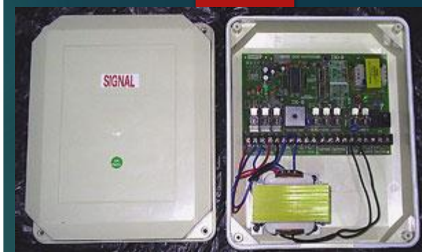
Computerised Control Panel
