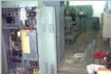
Working environment is very dangerous and hot, lots of moving parts and high voltages equipment are still in operation
