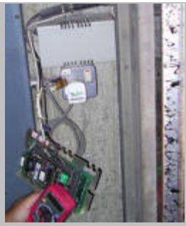
Power supply in lift shaft are inspected to ensure the voltage is enough to power the whole system
