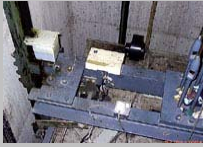
Inspection of lift car top preparation to install the Securitex Tele-elevator-control system.
