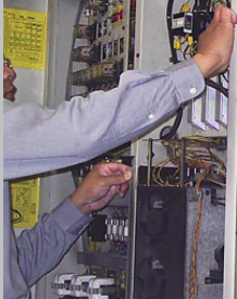
Management inspect elevator controller before interfacing of the tele-elevator-controller
