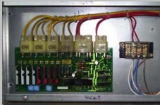
Cable termination and system installed in the lift motor room will be of manufacturer standard.
