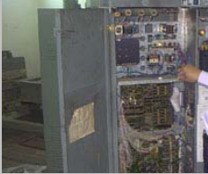
All final handover will be inspected by our highly trained system engineer and top management to ensure the newly installed elevator system do not interfere with the elevator operation
